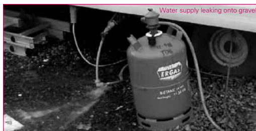
Water supply leaking onto gravel
